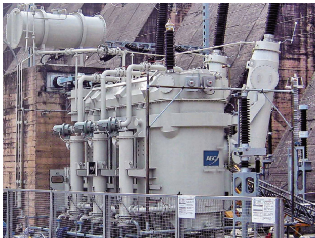
Fig. 2 Step-up transformer 112 MVA on H2 unit of HE „Bajina Basta“ manufactured by ABS Minel Transformatori Ripanj
